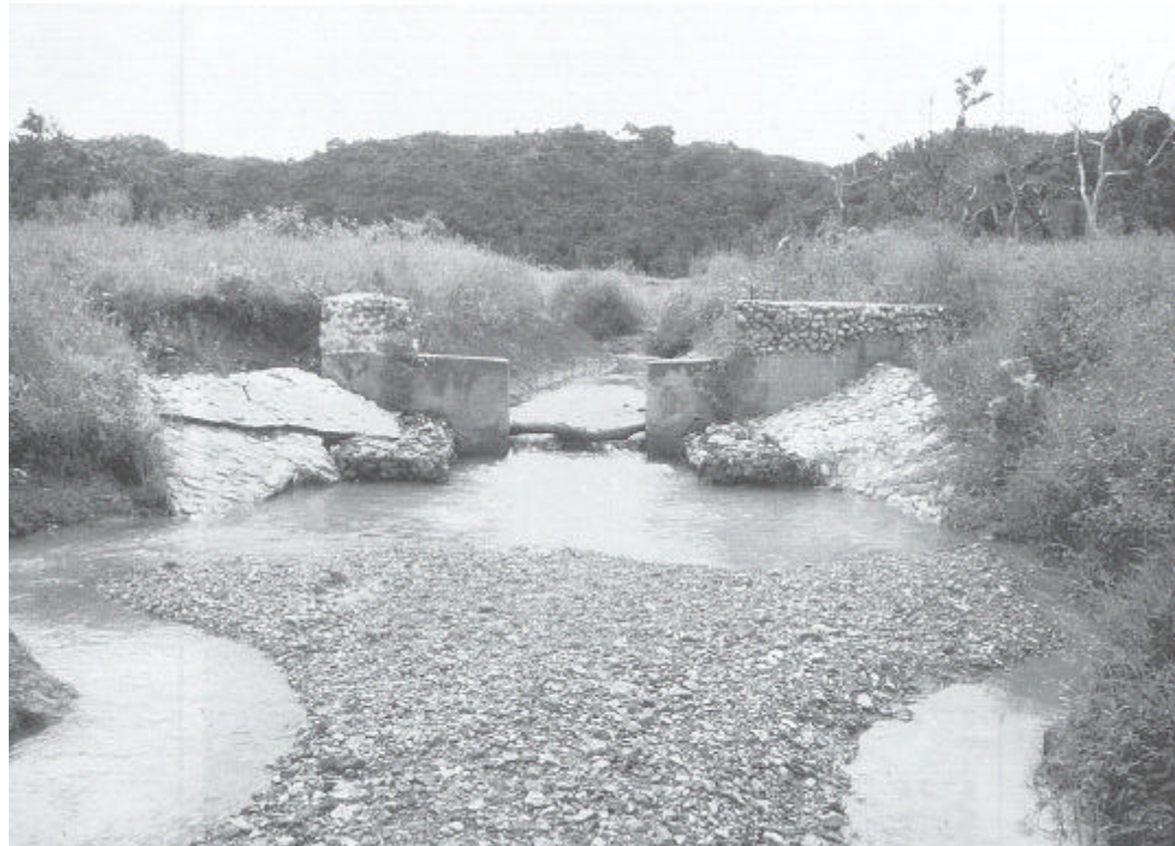
FIGURE 67 Scouring and sedimentation in a drop structure after a high discharge
