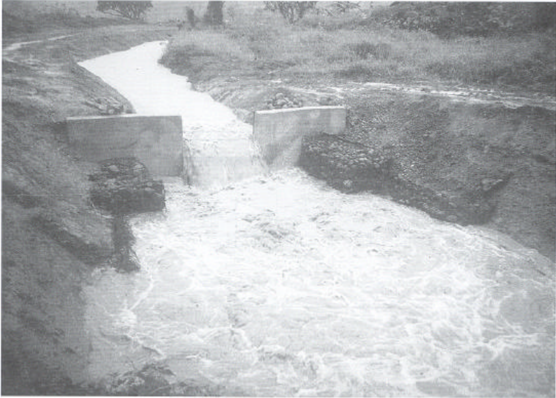
FIGURE 9 A main drain is often a canalized stream
